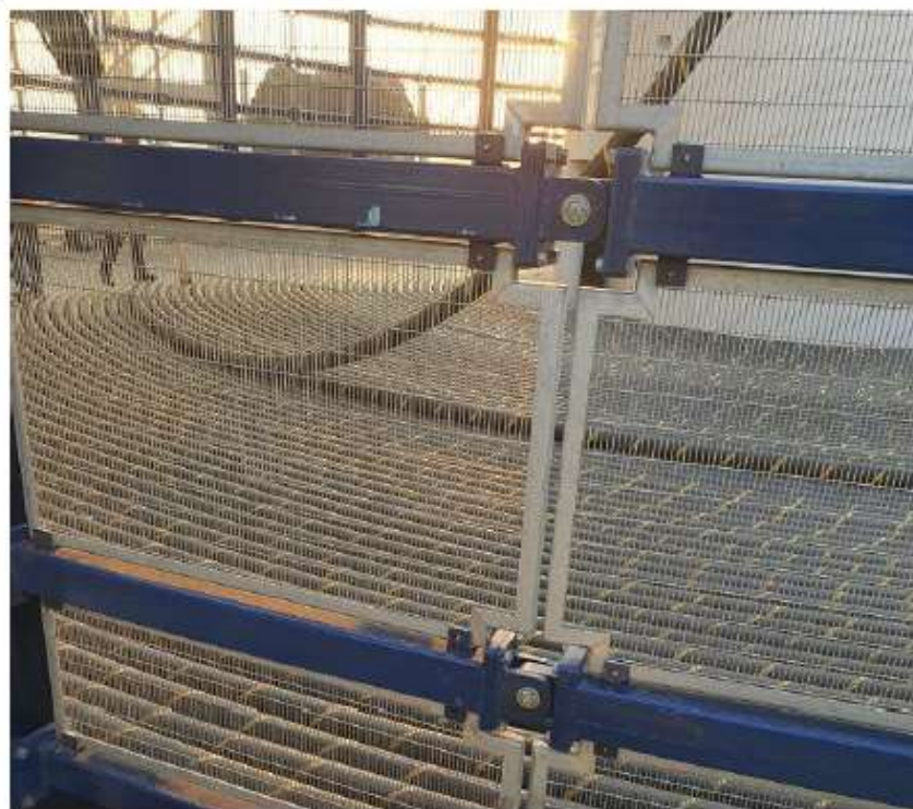
C2 HVDC Cable Load – LDV – Pole 1 stow in FWD Carousel.
