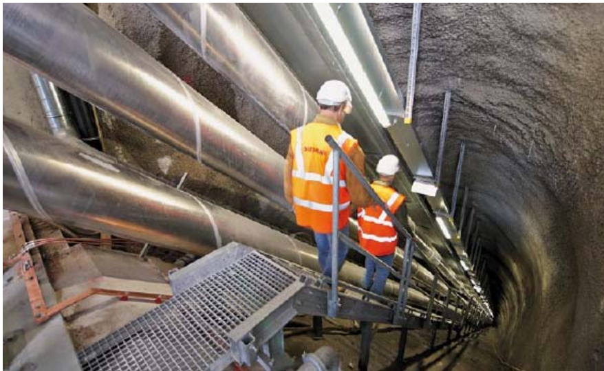
Figure 29: GILs installed in tunnels (SIEMENS).
