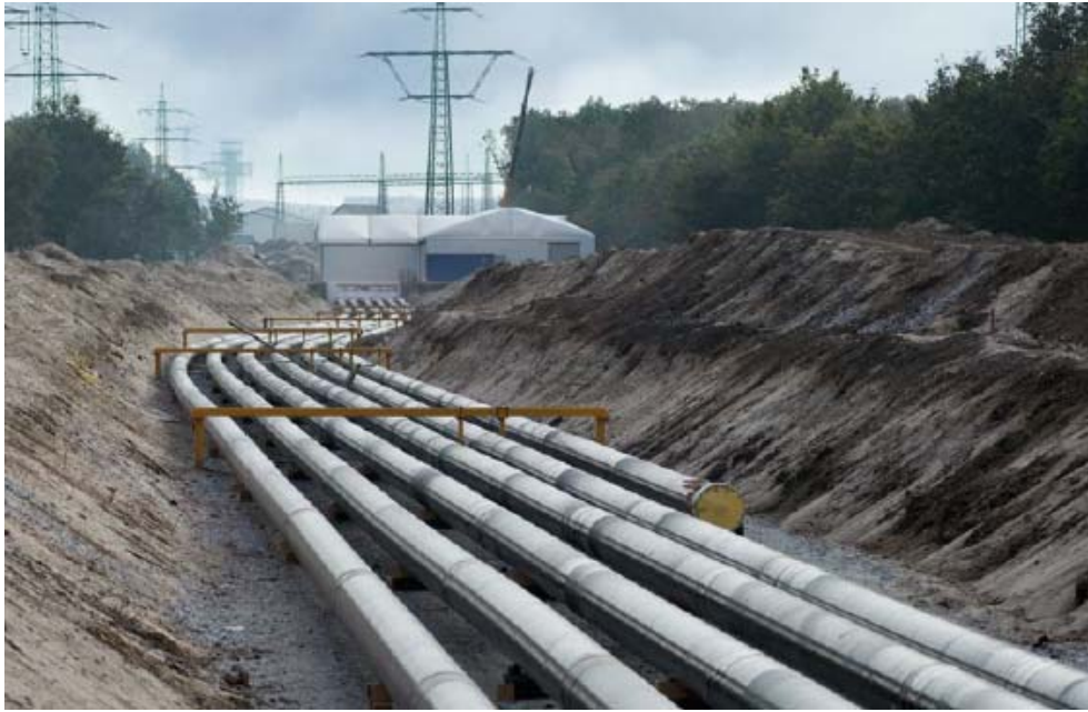
Figure 30: Double circuit GIL installation (Foto: SIEMENS).
