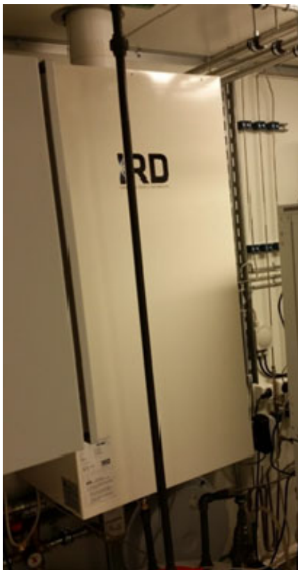
Figure 6. \mu\text{CHP} as wall installation.
