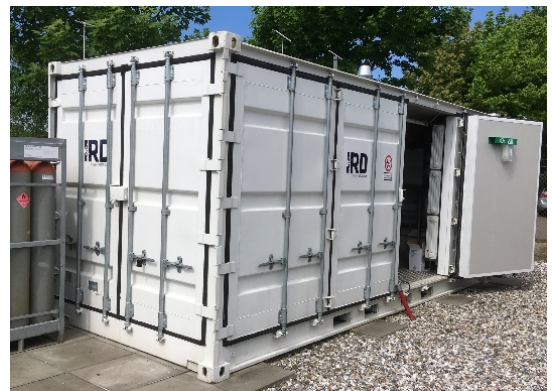
Figure 3. Insulated 20-ft container at M/R Helle in Varde.
