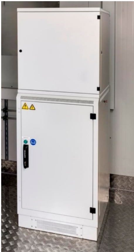
Figure 5. PEM electrolyser with drying system on top.
