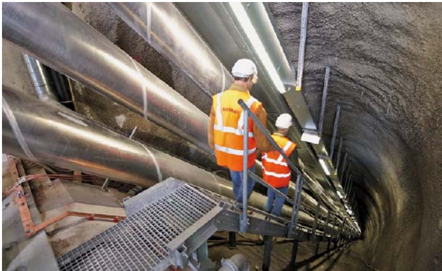
Figure 29: GILs installed in tunnels (SIEMENS).
