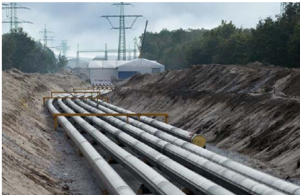
Figure 30: Double circuit GIL installation (Foto: SIEMENS).
