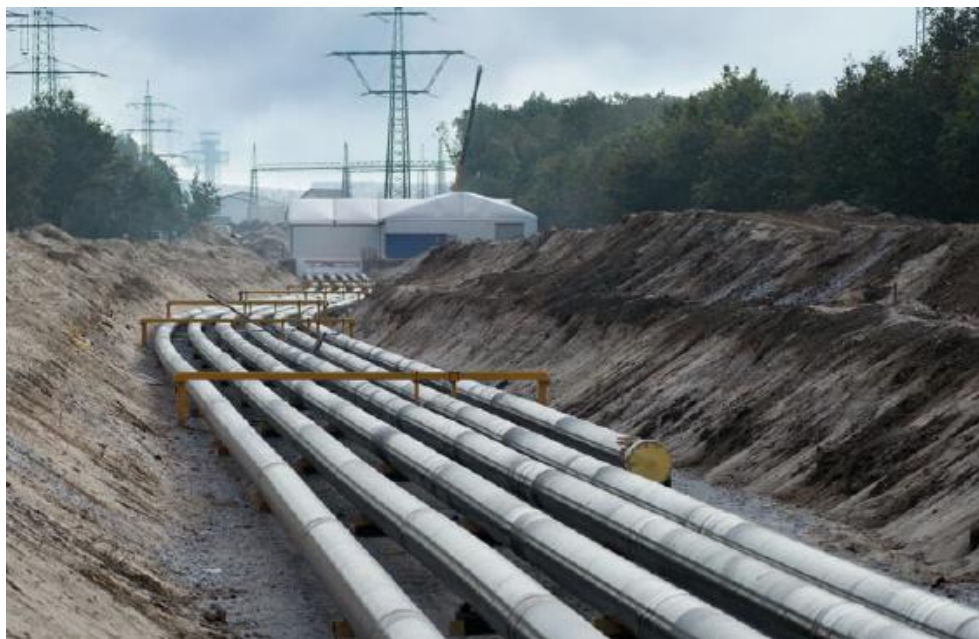
Figur 30 To-systems GIL-installation (Foto: Siemens).
